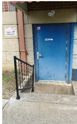
A stair rail has been added to the outside west entrance of Lions Hall.
