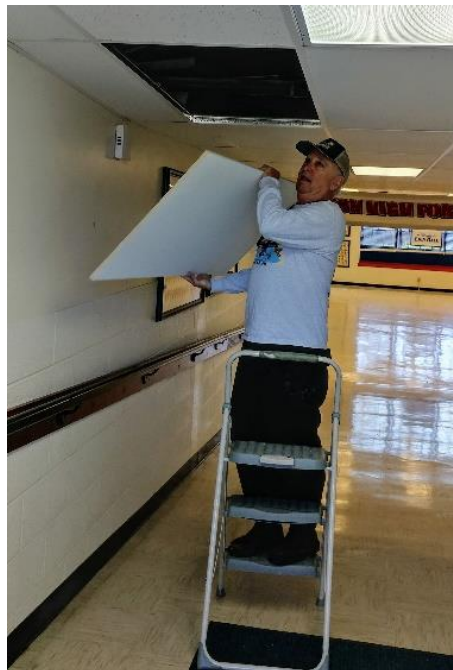
Damaged or stained ceiling tiles have been replaced. Shown is ILAA President Mickey Collier.
